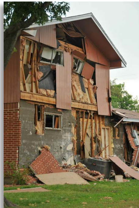
The shock from the deflagration of a fertilizer storage facility resulted in the damage to this single-family dwelling. (Federal Emergency Management Agency/Norman Lenburg)
